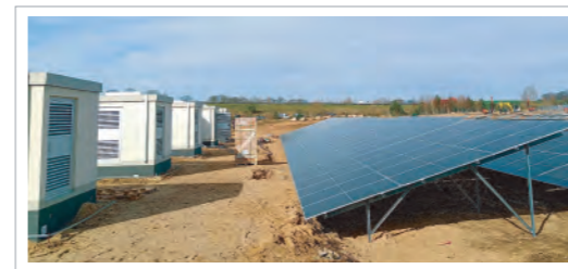
Germany 16.77MWh Containerized Energy Storage Project
