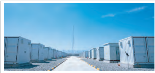
Jimusaer 150MWh Project
