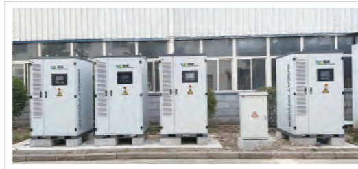
Zhumadian Zhongji Huajun 2.8MWh Project
