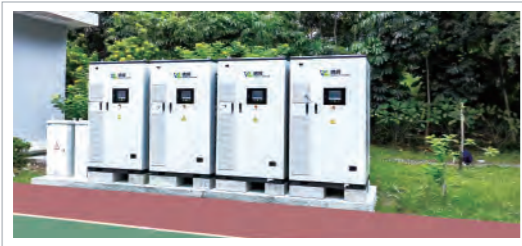
Shenzhen Yinghe 3.26MWh Project
