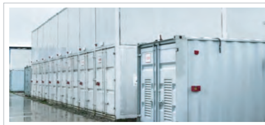
State-Owned Shipyard 100MWh Energy Storage Station Project
