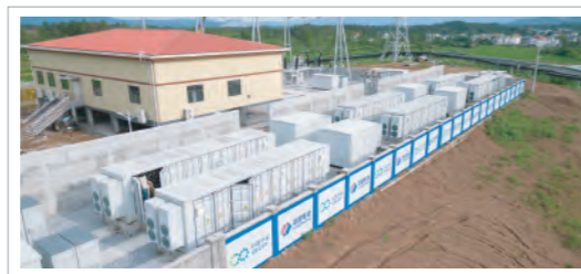
Ji'an 15MWh Agro-Photovoltaic Complementary Project
