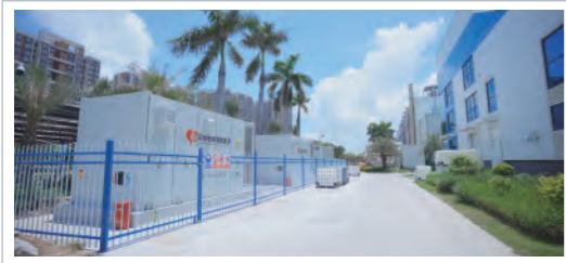
Zhuhai Great Power Production 29.77MWh Project
