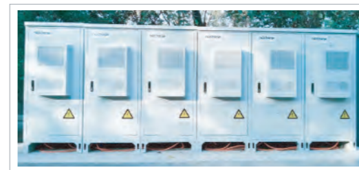
India 2MWh High-Grid Photovoltaic Storage Project
