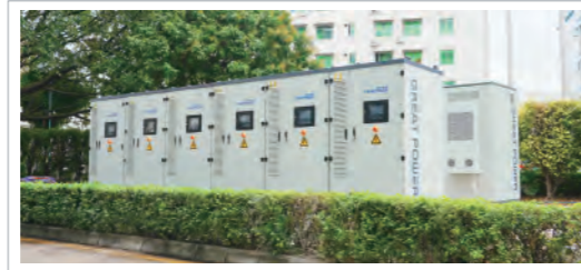
Guangzhou Production 7.33MWh Project
