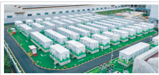
Nanning 100MWh Energy Storage Project
