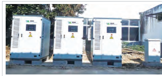
Runan Yuxin 1.5MWh Project
