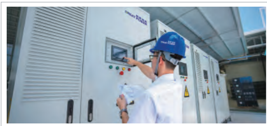
Guangzhou Xinli 2.33MWh Project
